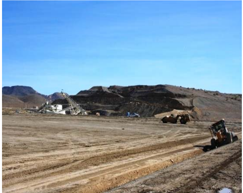
(Above) Grading work is completed at Relief Canyon's new heap leach pad.
