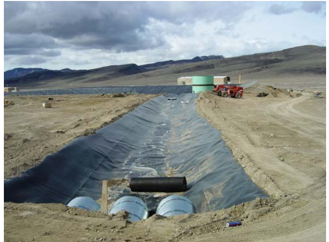
The secondary liner bed in which the fluid pipe is being laid
