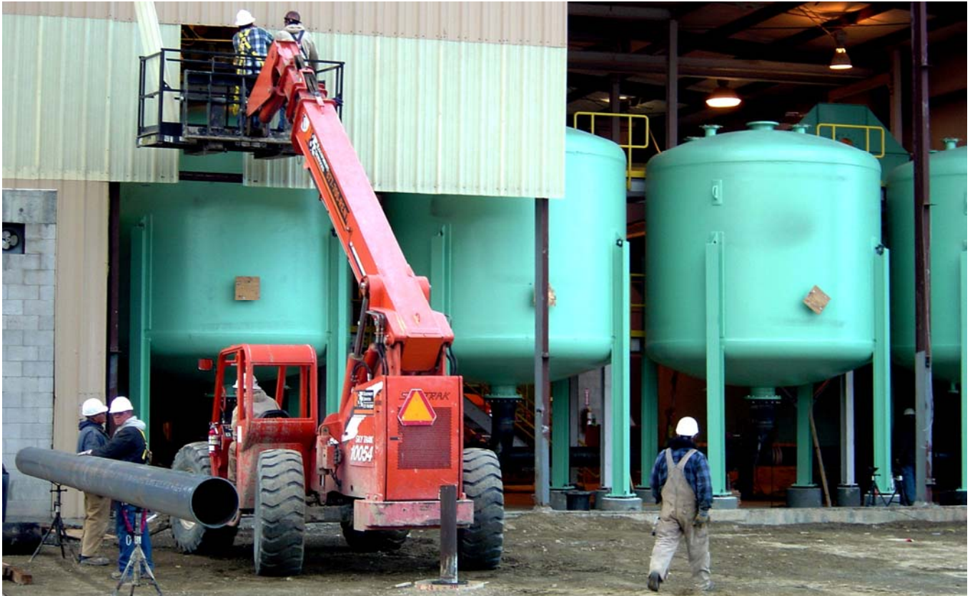
Crews work to reassemble the siding that was removed for the installation of FGC's pressure vessels (seen above).
