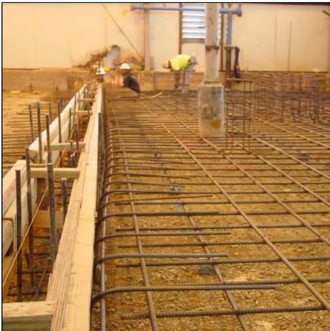
Plant construction is scheduled for December. Above, crews prepare to pour concrete.
