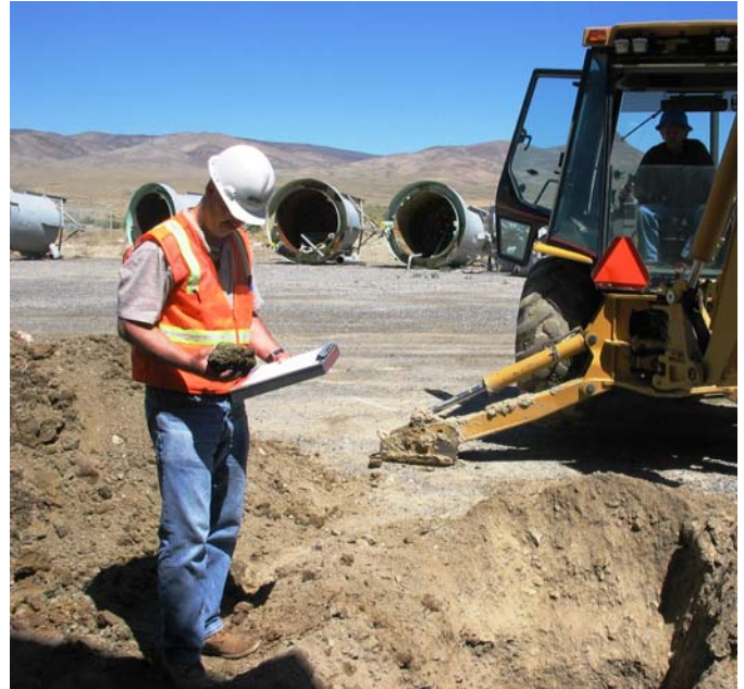
Kevin White of AMEC conducts a soil stability survey for plant construction.
