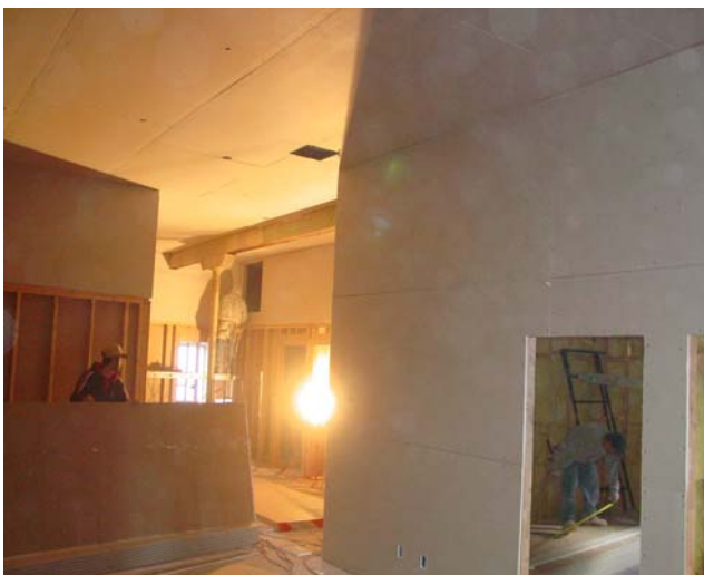
Firstgold Corp employees work to complete the final phase of sheet rock at the Lovelock, NV office.
