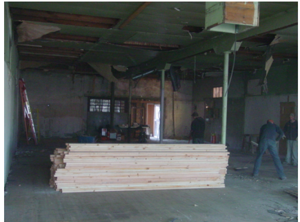
Firstgold Corp's new office in Lovelock, NV undergoing demo prior to improvement.
